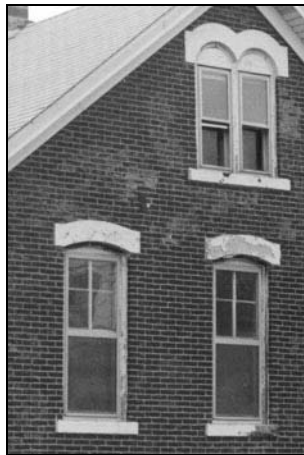
Figure 152: Detail, 2329 Washington, early lintel form
