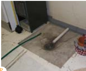
foundation drain to floor drain - IMPROPER
