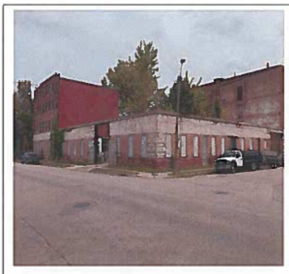
Remaining front and side walls of building torn down years ago. Window glazing positive on Elm St Windows North of wall opening to scrap yard.
