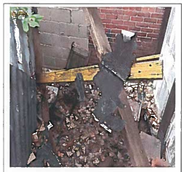
A-20/20A: Roofing debris throughout south portion of the building.
