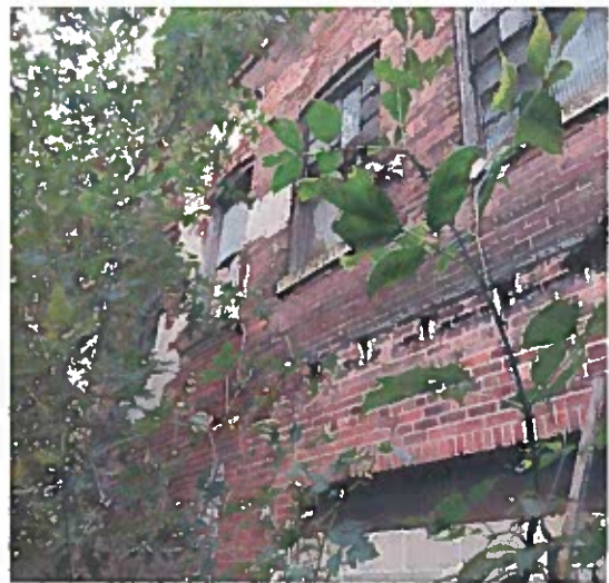
A-21/22: Flashing tar on Elm St. building from collapsed boiler building.
