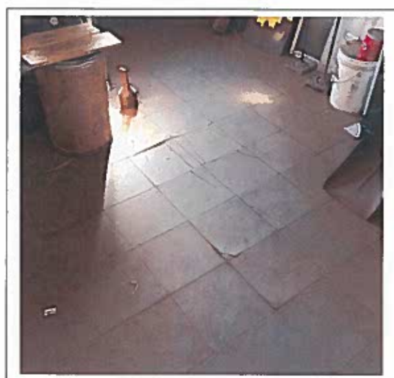
A-70, 71, 73: Industrial tile front office and entry. 9x9 floor tile under industrial tile positive also. Mastic associated with tile positive
