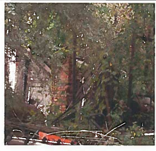
Building not inspected, Half collapsed and no access
