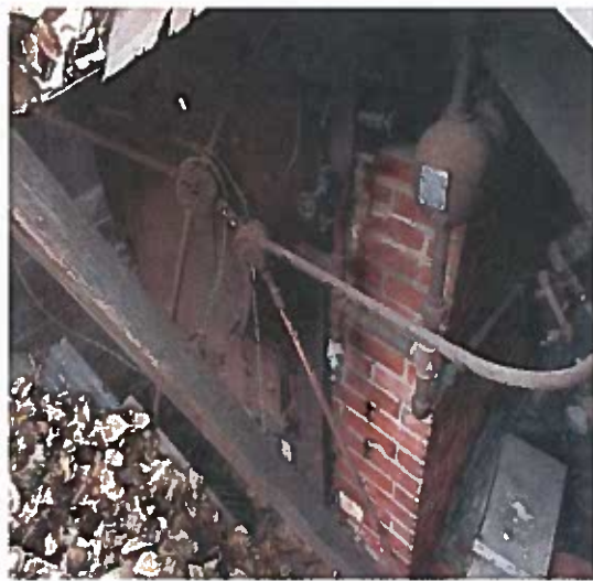
Boiler in building not inspected. Roof collapsed on top of boiler. Will need to be inspected prior to demolition
