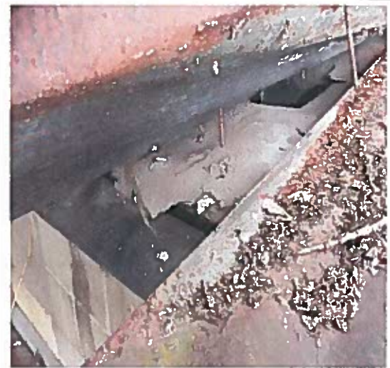
A-23: Tar paper from north section of collapsed building with boiler.
