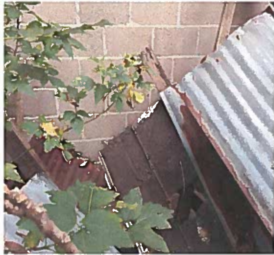
A-20/20A: Roofing debris from south portion of building
