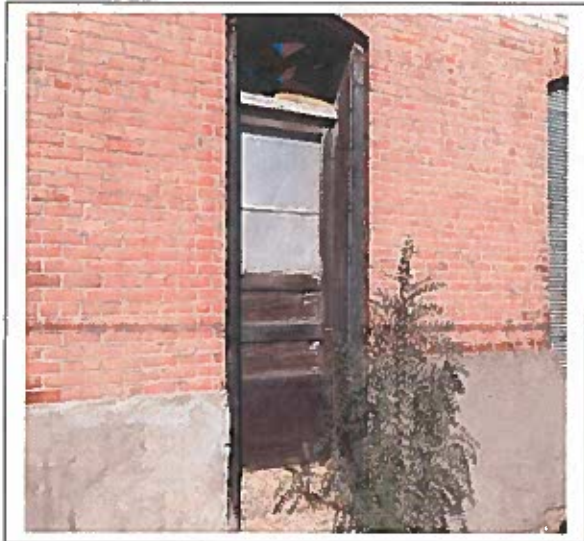
A-9: Caulking around Elm St. door, wood frame to brick.
