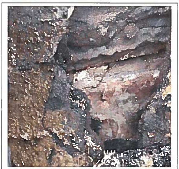
A-51: Flashing, parapet walls Elm St. building. A=54: Tar above flashing on parapet wall.
