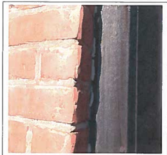
A-9 Caulking around Elm St. door, close up picture.
