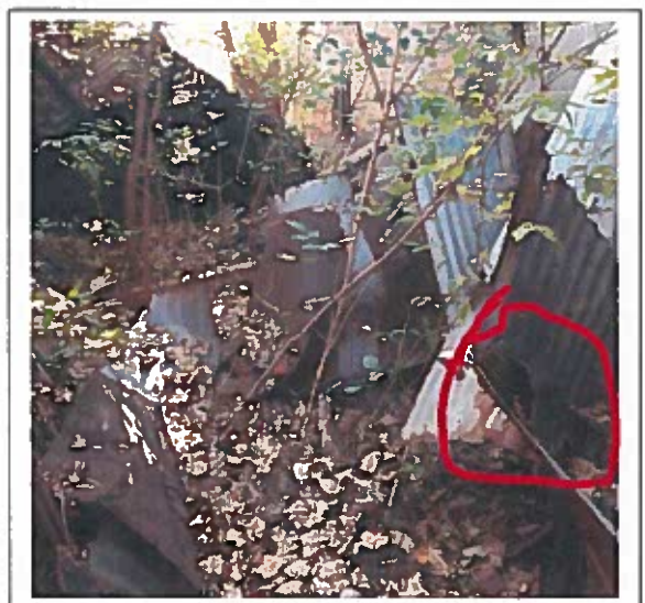
A-20/20A: Roof on south portion of boiler building. Debris throughout area.
