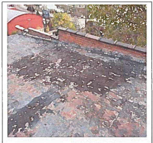
A-31, 32, 33, 35: Tar on metal roof, Elm st building.
