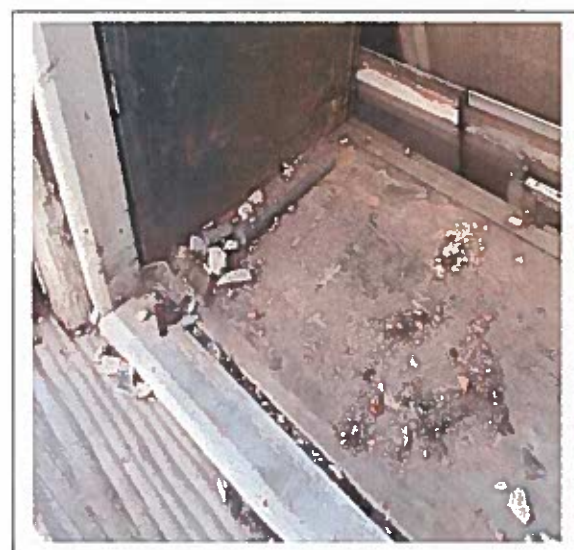
A-3: Window glazing debris in window sills of collapsed building. Windows gone except one window.
