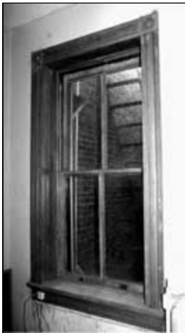
Following the relatively simple repairs, the window is weathertight, like new in appearance, and serviceable for many years to come. Photo: NPS files.
