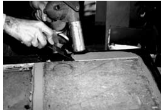
Sash can be removed and repaired in a convenient work area. Paint is being removed from this sash with a hot air gun. Photo: NPS files.
