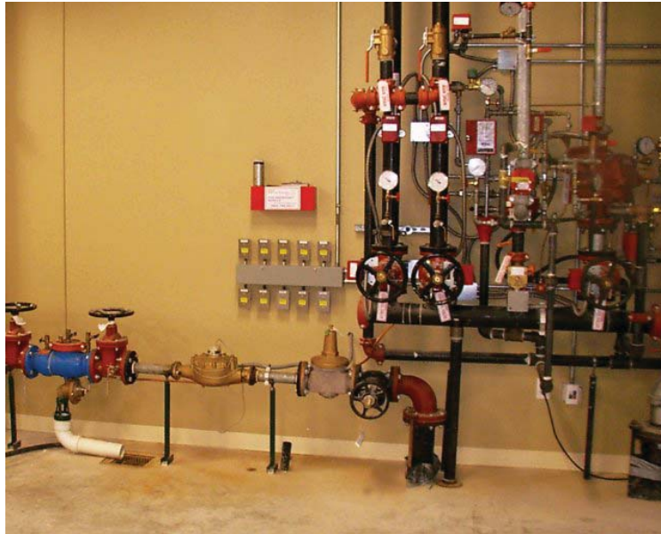
Typical Meter/Fire Sprinkler Room
